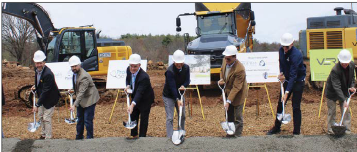
Brian M. Johnson ProHealth Physicians executives and city leaders break ground on the company's medical building on Farmington Avenue Friday.
